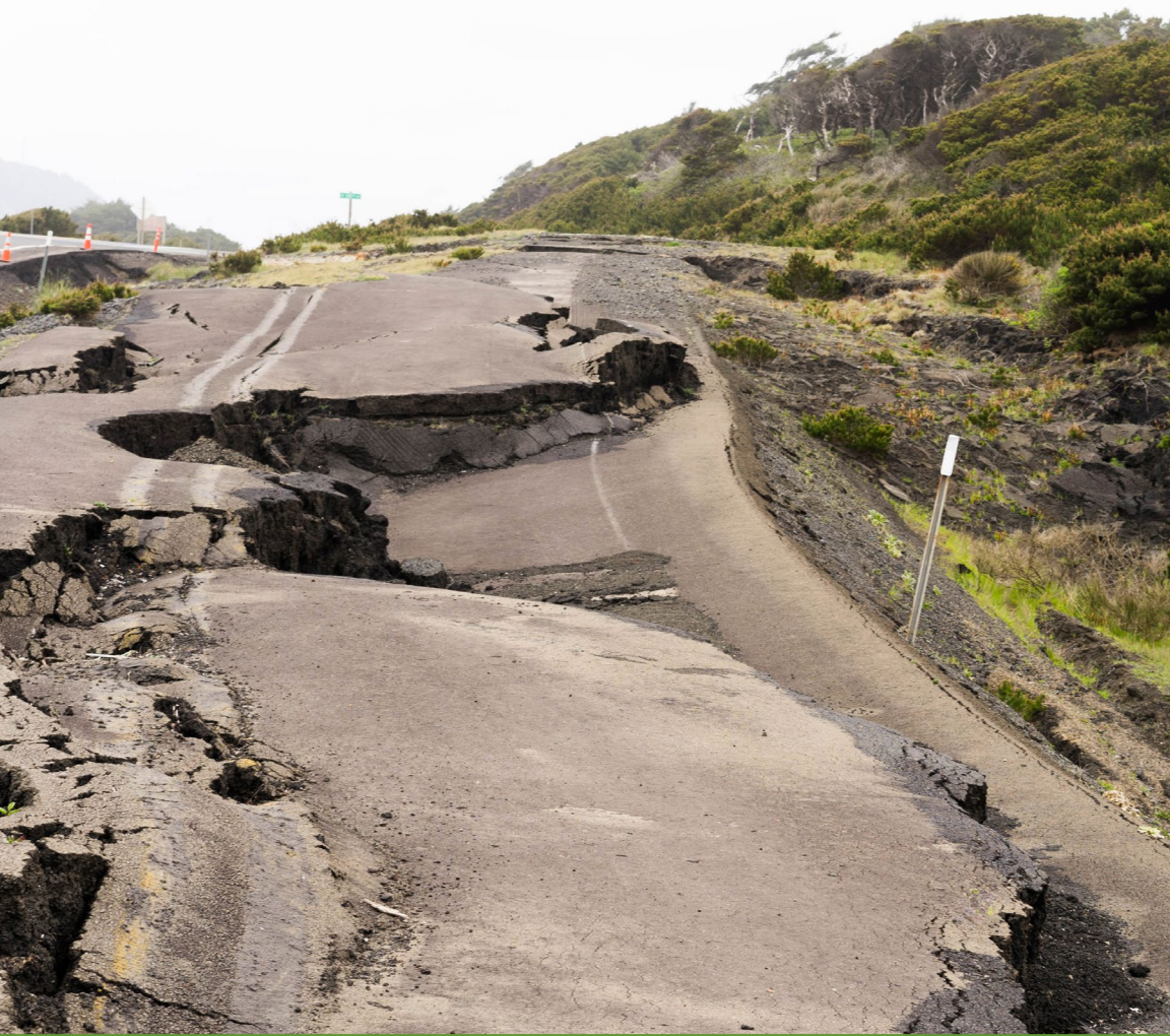
Photo description: Road buckled and damaged by earthquake.
